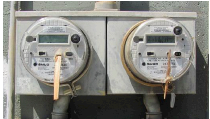
Figure 1 – Example of Attempted Power Theft
